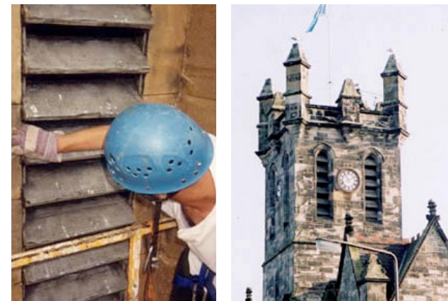
Louvre replaced on a listed building with radio transparent replica Photographs courtesy of Dynamic Concepts
