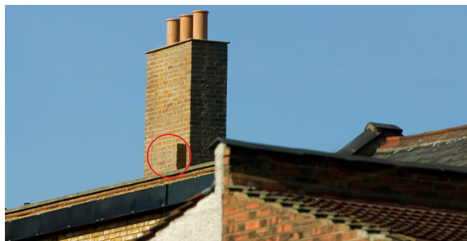
Good example of disguised equipment
