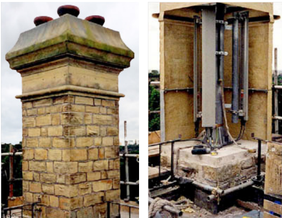
Replica chimney housing equipment Photographs courtesy of Dynamic Concepts
